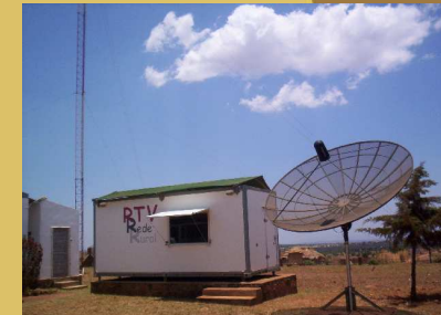
VSATs could be set up at all regional offices to increase coverage
